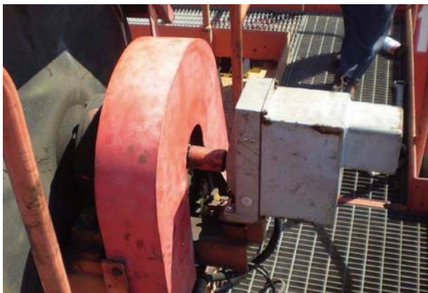
Mechanical cam limit switch for position monitoring at the hoist of a RTG crane.
