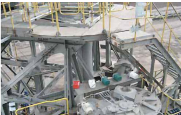
Before: Frame construction for the slewing gear between the superstructure and substructure of the excavator with several mechanical cam limit switches for position monitoring.
